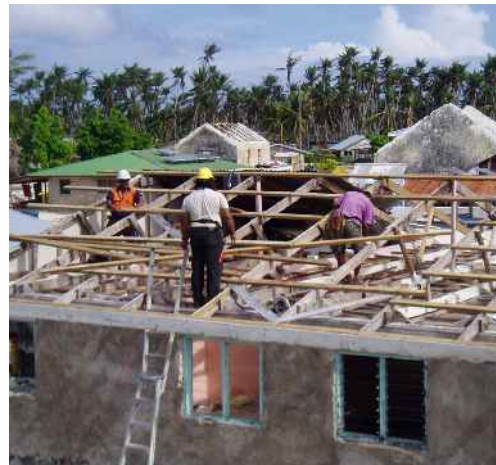
Recovery after the TC Percy 2005 in Pukapuka
