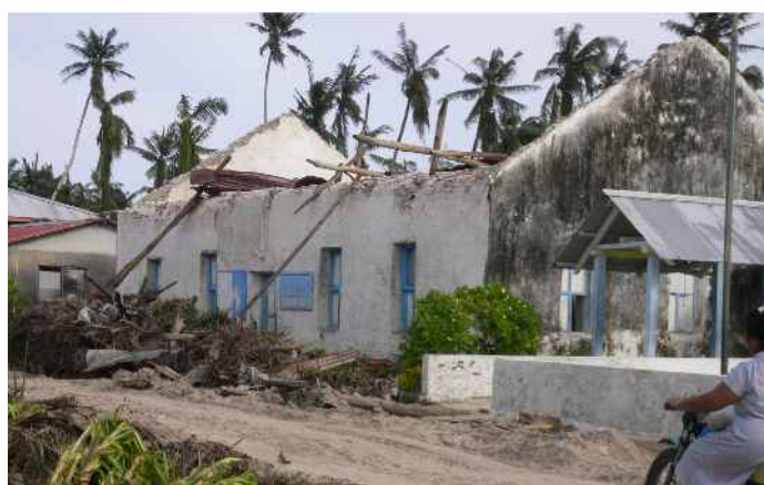
Damaged building in Pukapuka after TC Sally 2005
