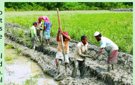
Community members from Char Kukri Mukri build mounds for protective and productive plantations, Bhola District, Bangladesh
